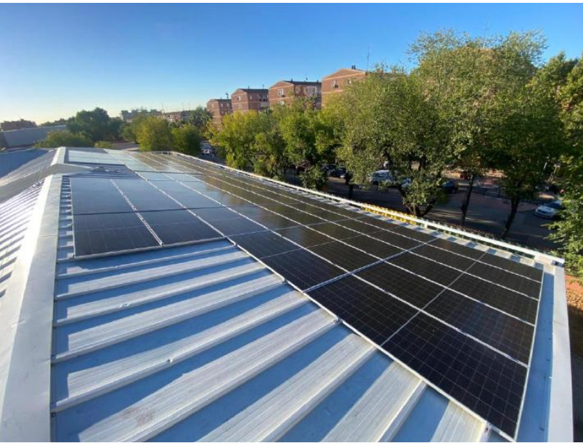
The energy community's first municipal installation on the Civic Centre Las Margaritas (40 kWp) © Getafe
